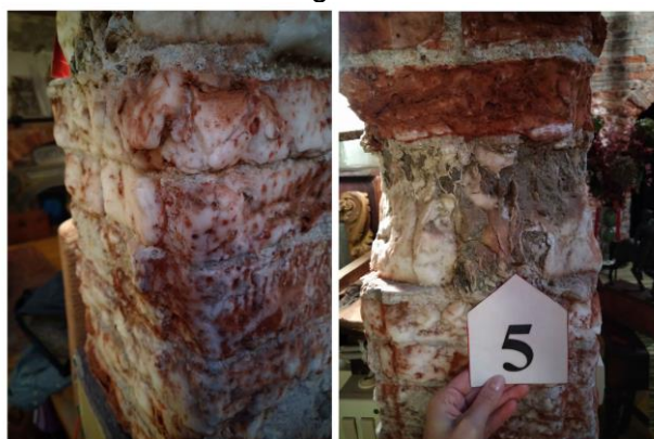
Figure 1. Efflorescence and loss of material on masonry.
